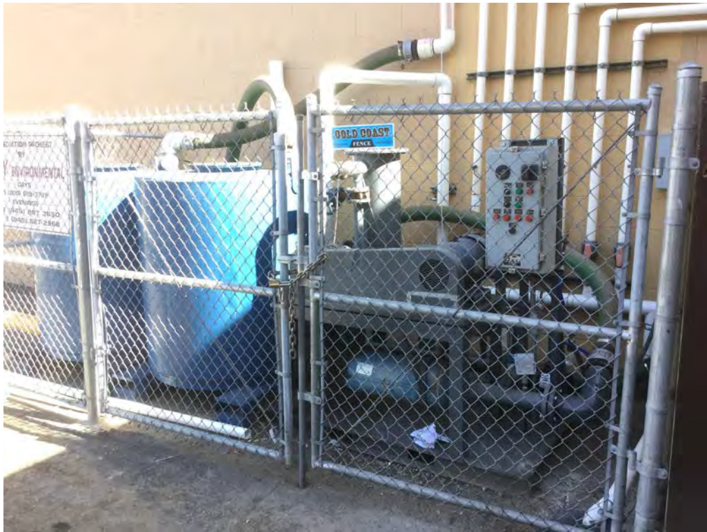
Vapor extraction system at rear of former Granada Hills Cleaners location. 16233 San Fernando Mission Blvd., Granada Hills, 91344
