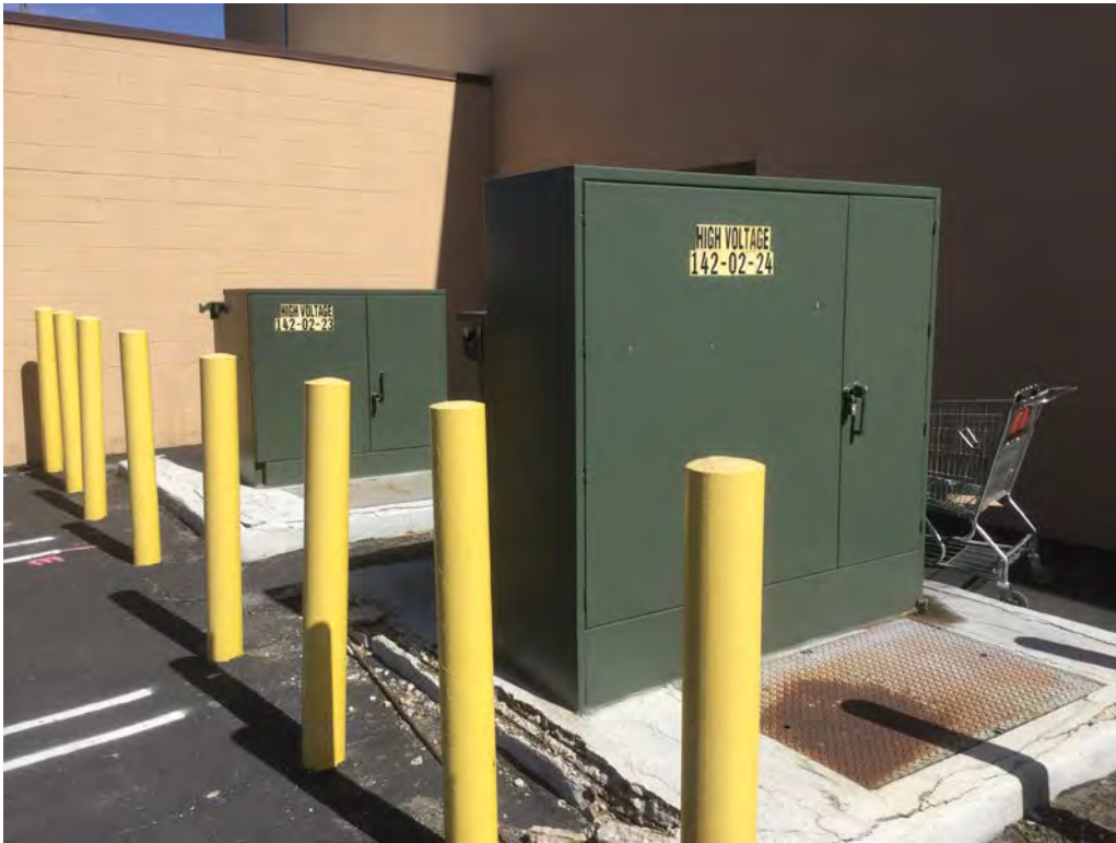
Vaulted transformers on the subject property. 16201 – 16287 San Fernando Mission Blvd., Granada Hills, 91344
